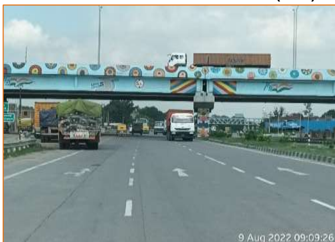
Pavement Condition at km. 782+500 (RHS)
