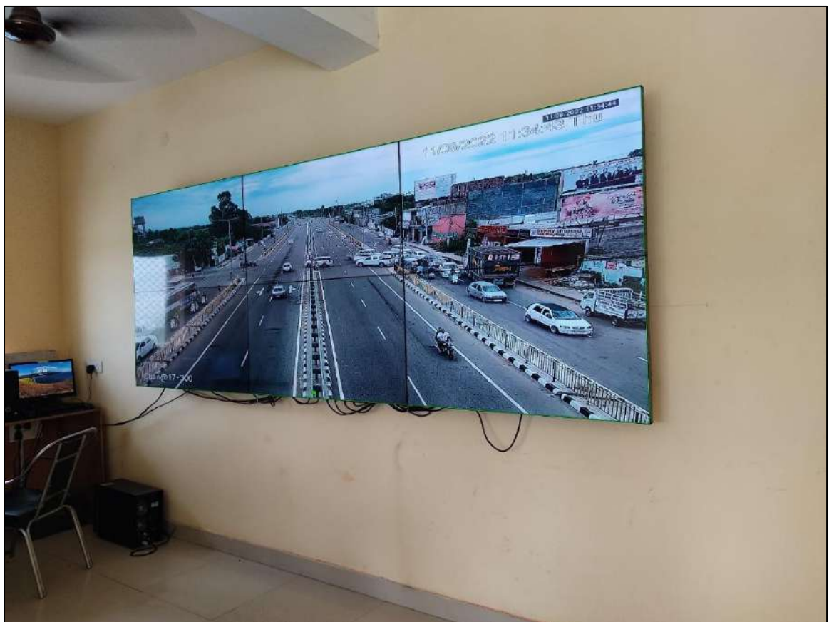
Figure 9-18 Video wall at HTMS Control room
