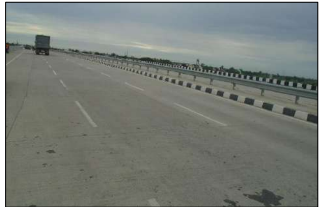
Crash Barrier at curve location
