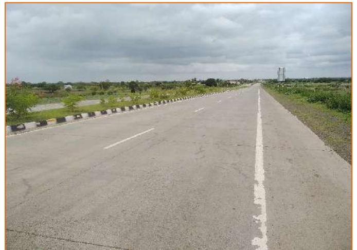
Pavement Condition at km. 319+100 (RHS)
