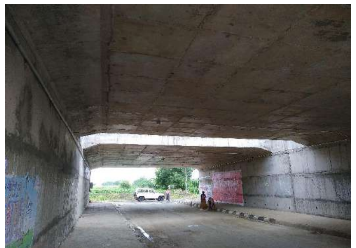
Lighting arrangement made under structures
