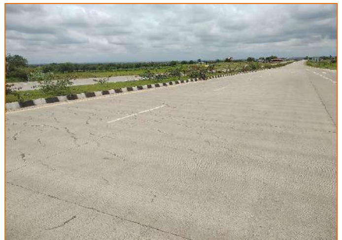
Pavement Condition at km. 304+600 (LHS)
