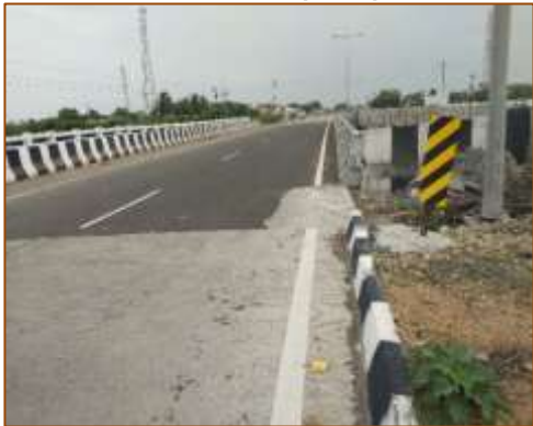
Side View of Minor Bridge at km. 450+241 (LHS) - New - Approach settled
