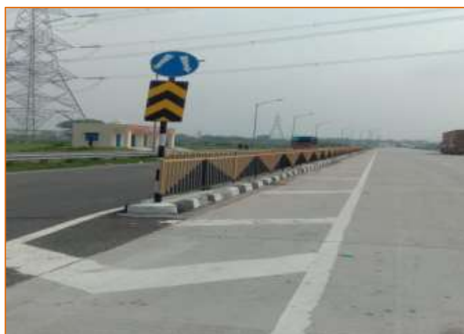
Pedestrian Guard Rail at km.766+600
