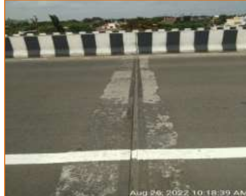
Filled expansion joint of Flyover at km. 130.650 (RHS)
