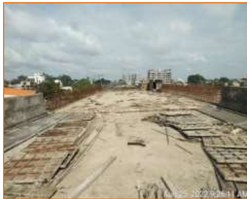
Expansion joint & crash barrier of Flyover is in progress at km. 136.857 (BHS)
