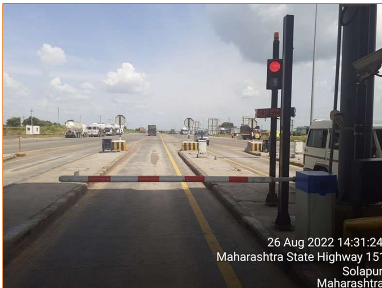
Figure 9-4 Automatic Lane Barrier
