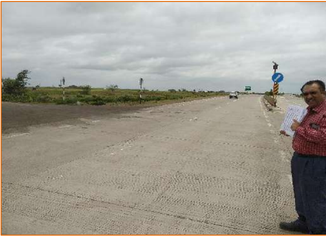
Pavement Condition at km. 306+500 (LHS)
