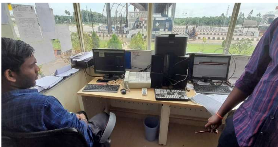
Figure 9-14 Work Stations at Control room
