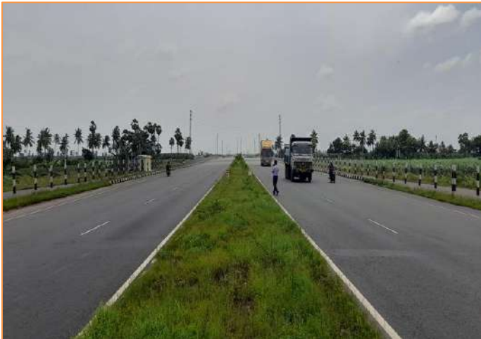
Pavement Condition at km. 41+200
