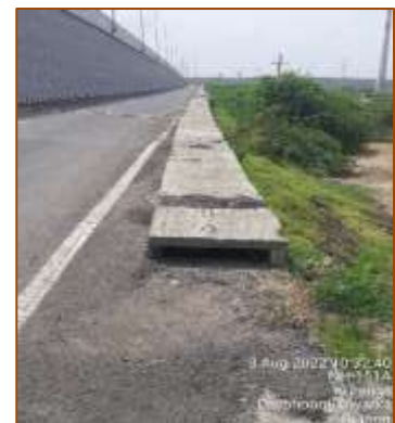
Built-up drain from km. 467+601 to km. 468+347 (LHS)
