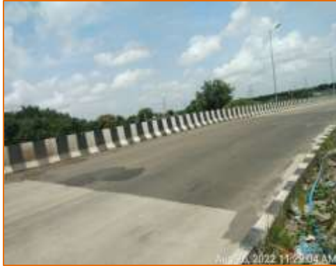
LVUP at km. 114.080 (LHS)
