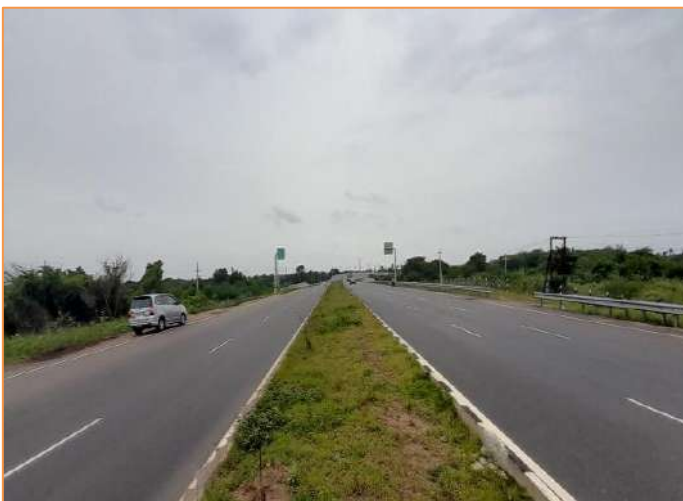
Pavement Condition at km. 55+100
