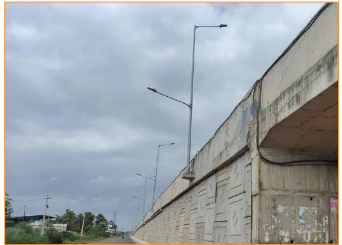
Highway Lighting at km. 44+135
