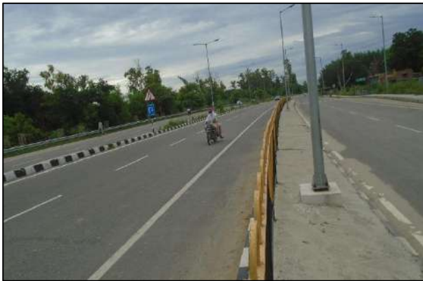
Pedestrian Guard Rail at km. 69+400
