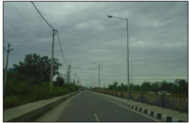
Street Lighting at Service Road
