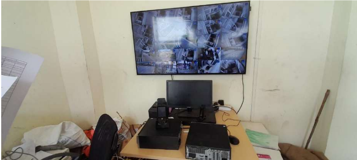
Figure 9-13 CCTV screen at the Toll Plaza Control Room
