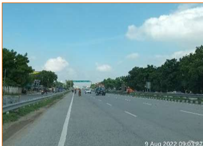
Pavement Condition at km. 785+200 (RHS)
