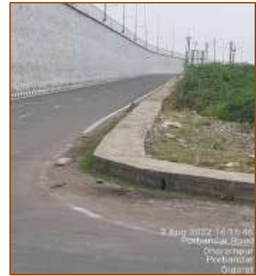
Built-up drain from km. 390+170 to km. 390+953 (LHS)
