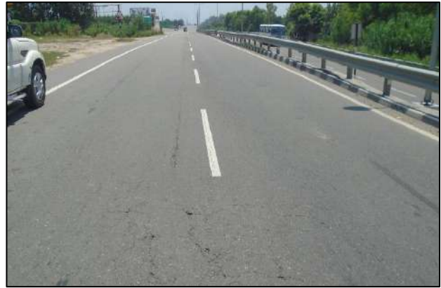
Pavement Condition at km. 59+000
