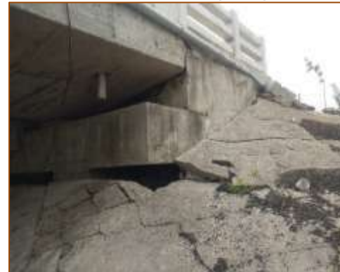
Settled CC Pitching at A1 side of MJB at km. 422+314 (LHS)
