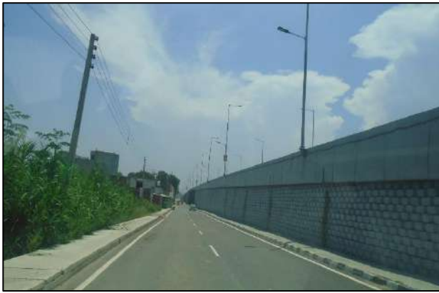
Street Lighting at Structure Approach
