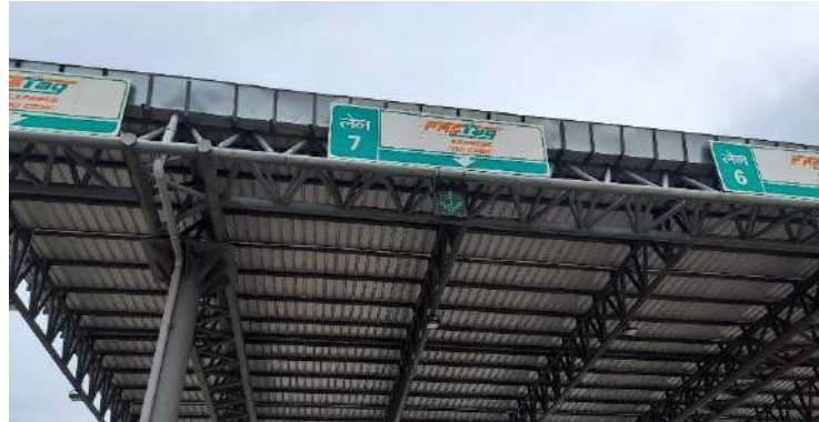
Figure 9-9 Over Head Lane Signal (OHLS)
