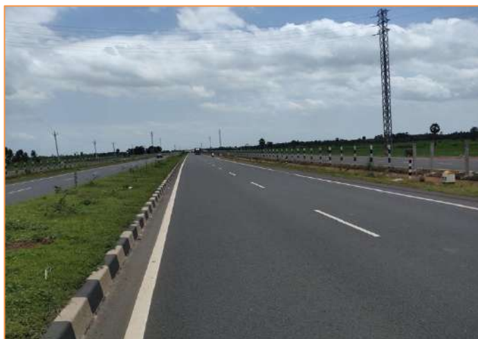
Pavement Condition at km. 71+300
