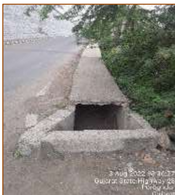
Built-up drain from km. 400+319 to km. 400+700 (LHS)
