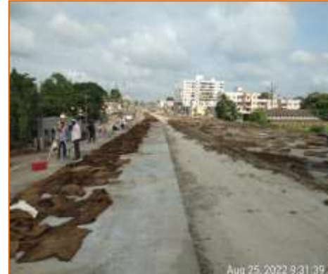
DLC & PQC of Flyover is in progress at km. 136.857 @ Solapur side (BHS)
