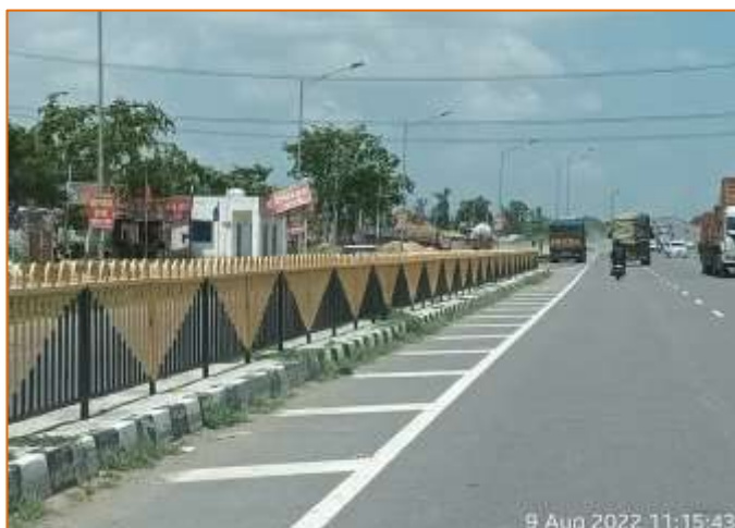
Pedestrian Guard Rail at km. 727+900
