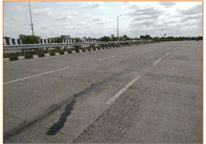
Pavement Condition at km. 287+700 (RHS)
