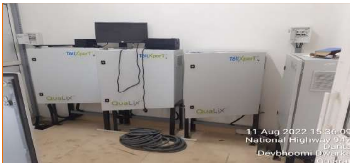
Figure 8-3 Lane Controllers for normal ETC lanes
