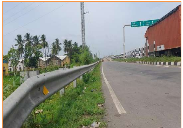
W beam Crash Barrier at km. 85+204
