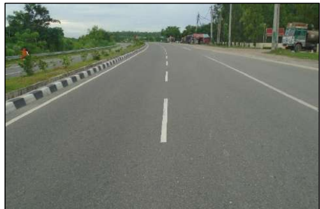
Pavement Condition at km.75+000
