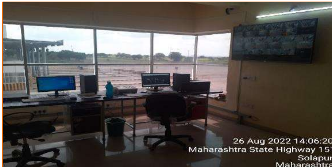
Figure 9-10 Incident Management Workstation at Control room
