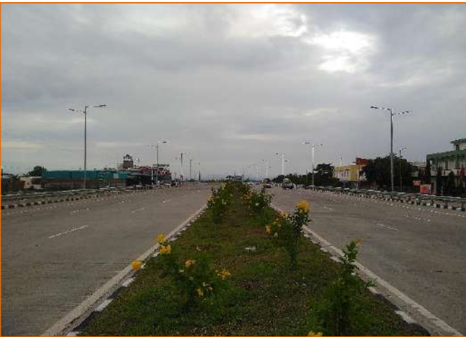
Pavement Condition at km. 285+750 (BHS)
