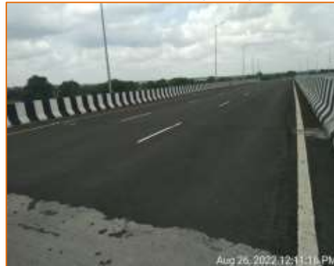
BC surface of Flyover at km. 102.700 (LHS)
