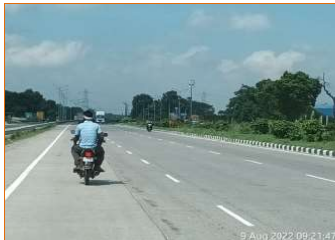
Pavement Condition at km. 785+650 (RHS)
