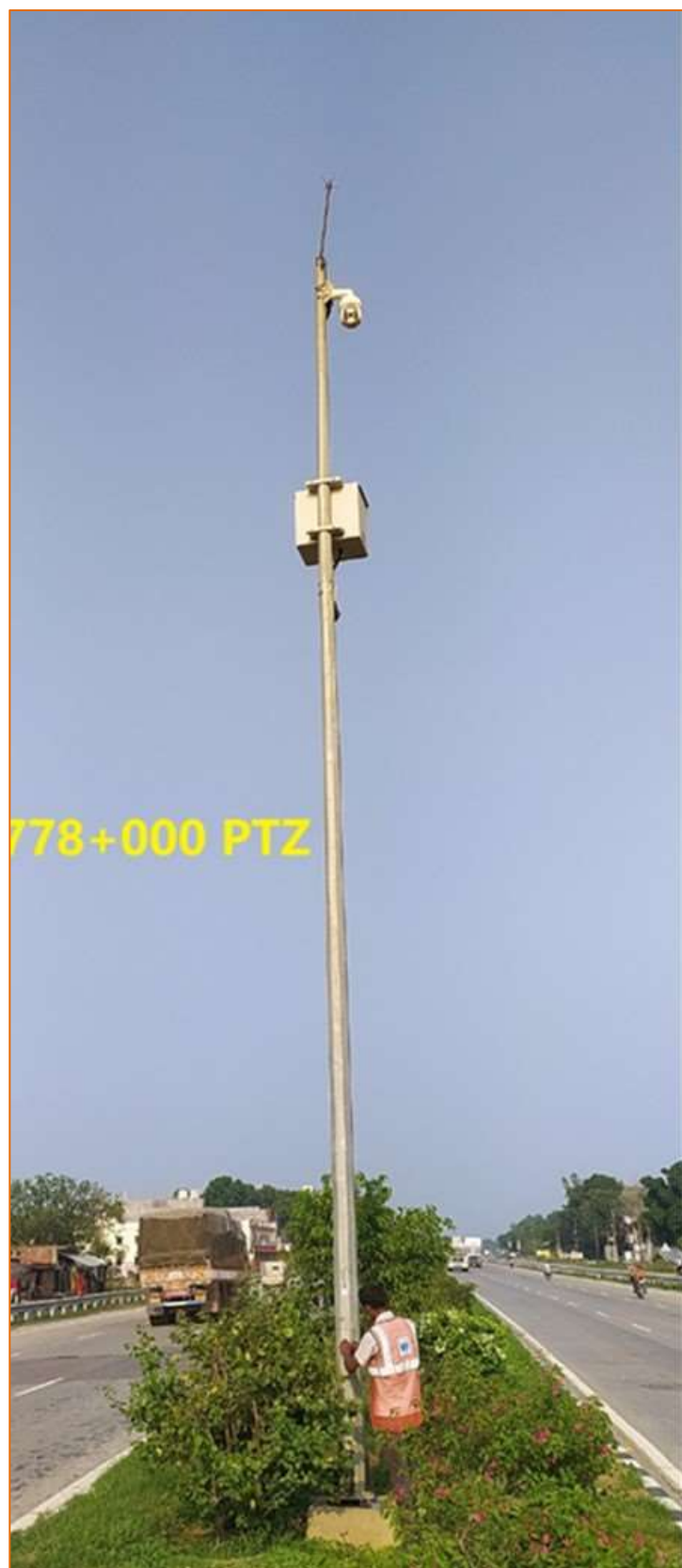
Figure 9-9 PTZ camera at km. 778.000
