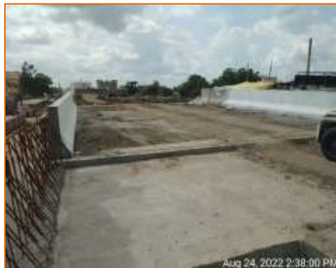
Wearing coat & Crash barrier of PUP pending at km. 136.657 (BHS)
