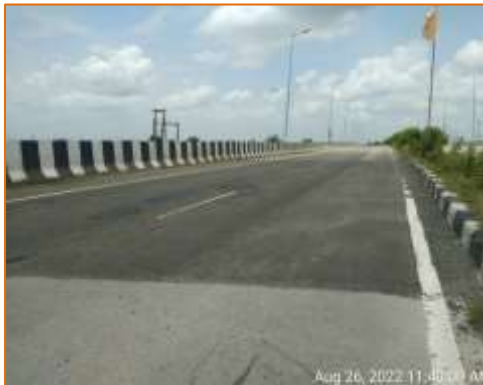
LVUP at km. 111.260 (LHS)
