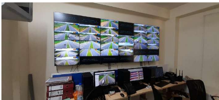
Figure 9-17 Video wall at ATMS Control room
