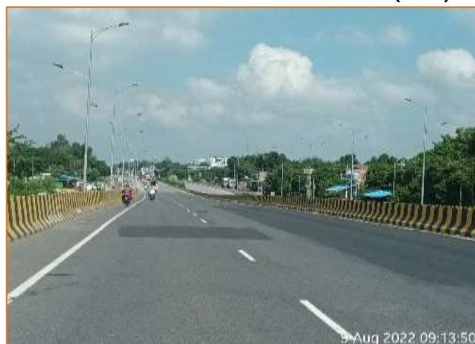
Pavement Condition at km. 779+600 (RHS)
