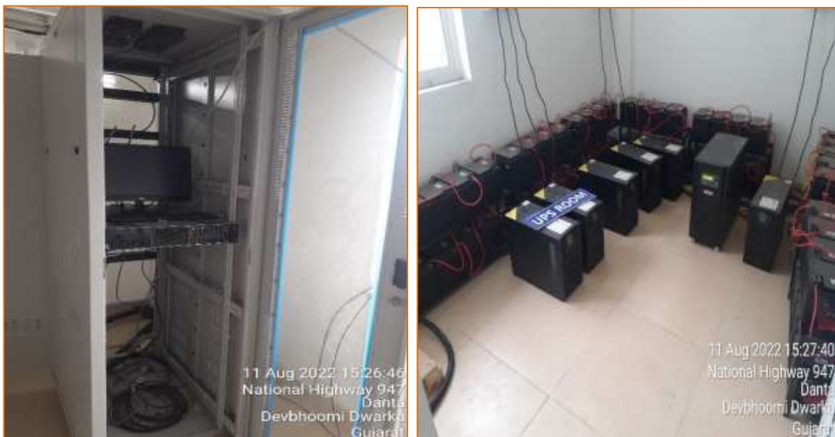
Figure 8-8 Control Room Equipment - Server & Switch rack/UPS Room
